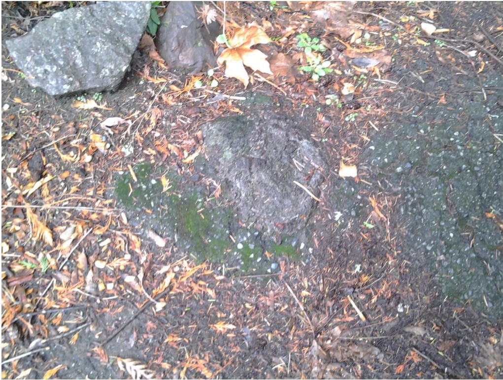
Figure 3. Photo of large root knotting up under driveway
